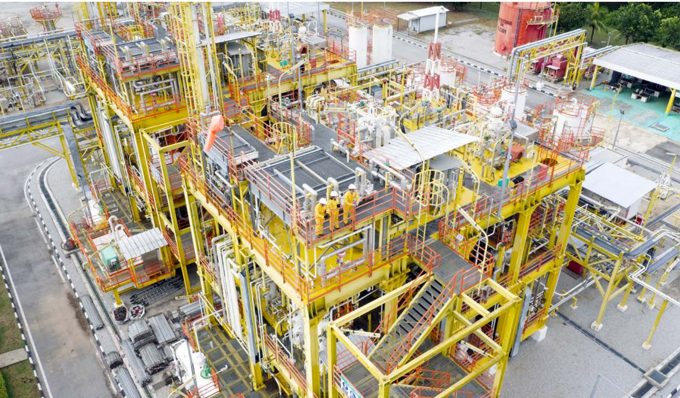
The Upstream Downstream Training Plant at INSTEP provides real plant experiential learning in a safe environment.
